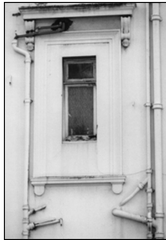
Excessive pipework (and inappropriate window) spoil this building
